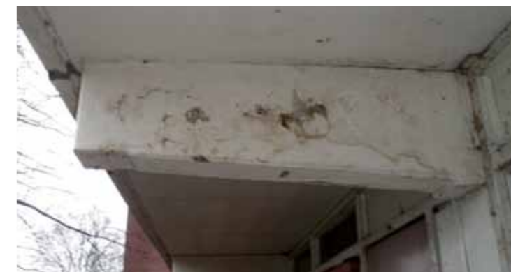
Brackets in which cracks were found during the visual inspection.
