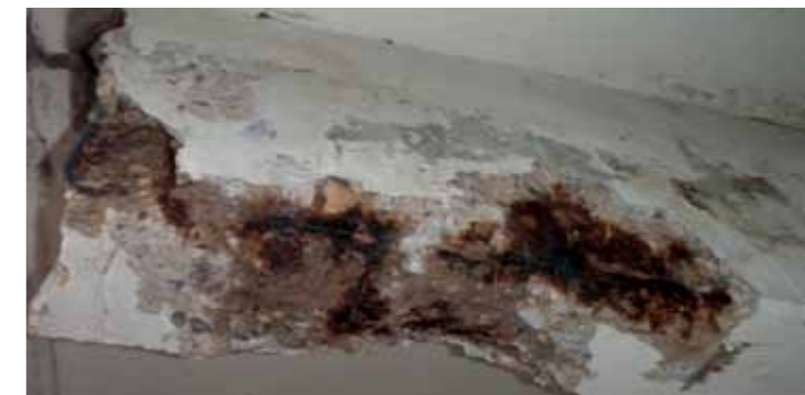
Serious reinforcing corrosion (initial chloride) found by destructive testing.
